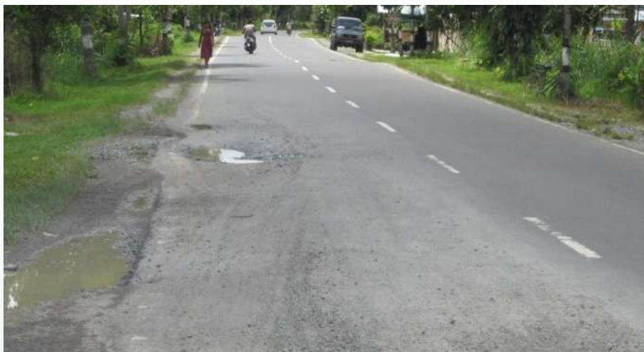
Gambar 4.8 Kondisi Akses Jalan menuju rencana lokasi pabrik Figure 4.8 Road access conditions to the planned factory location
