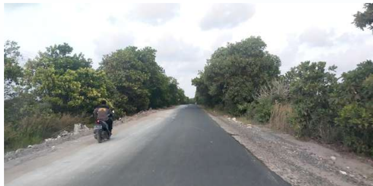
Gambar 4.17 Kondisi jalan poros Sukamara – Pantai Lunci – Jelai Figure 4.17 Condition of the Sukamara – Lunci Beach – Jelai axis road
